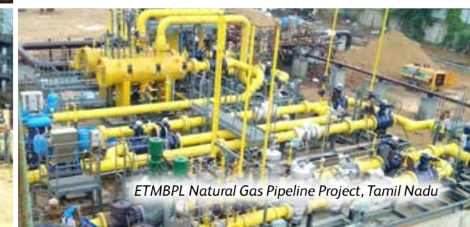
IOCL station piping, Ennore, Tamil Nadu
